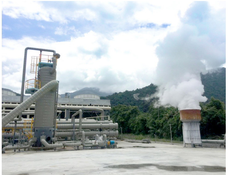
Quingshui geothermal plant, Taiwan (source: Shou-cheng Wang)
